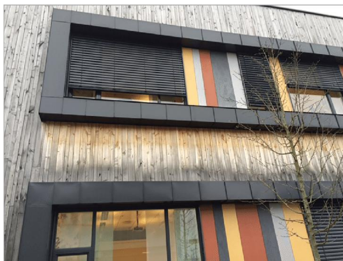
Figure 2: Unevenly weather exposed wood facade
