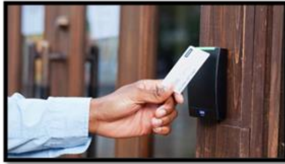
Figure 19: Card access control
