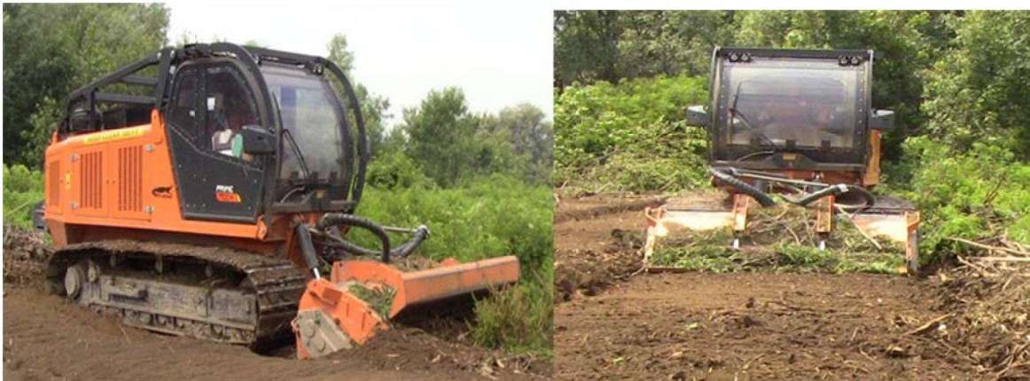
Figure 1: Site preparation of a poplar clearing with tracked self-propelled unit PT-400 equipped with multifunctional forestry tiller FAE 300/S-225
